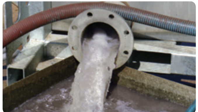
Fig 4. Filtrate being discharged from the Z300A unit.
